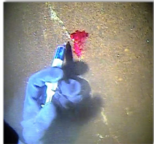
Figure 1 - Dye Used to Observe Leaks
